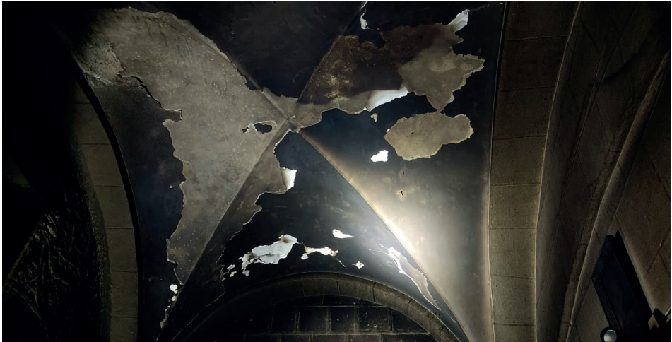
5. Damage to sacristy © TSC/UGRECYL Territorial Cell
