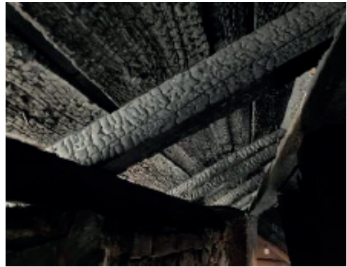
2. Roof after the fire © Peter Konečný
