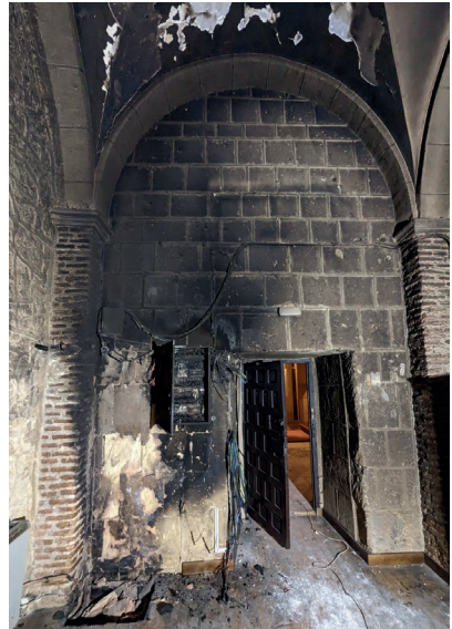
2. Origin of the fire: the electrical panel © TSC/UGRECYL Territorial Cell
